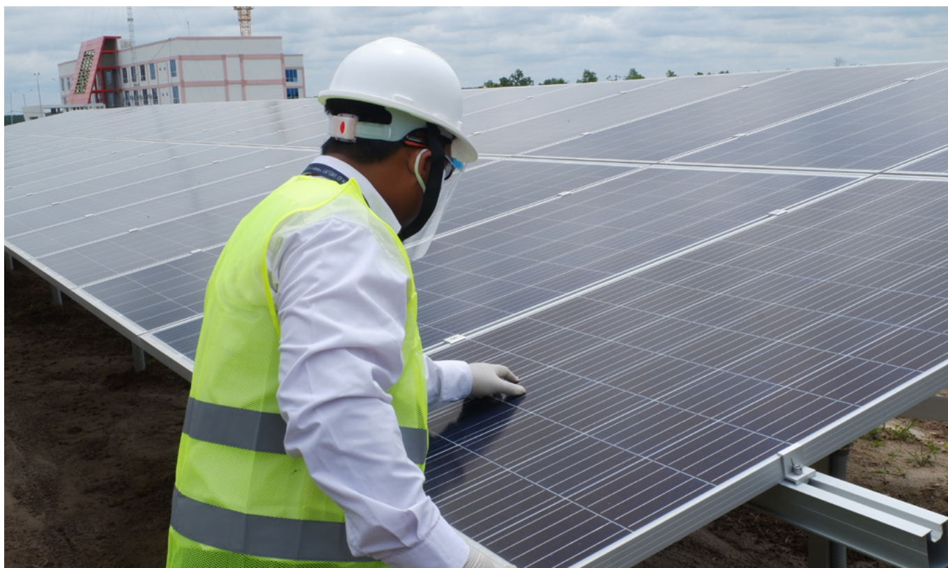
▲ An engineer at the Itera Campus solar power plant in Lampung Province, Sumatra
